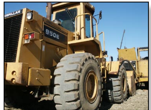
Grading has begun on Village Walk Plaza and Village Walk Murrieta Senior Apartments.
